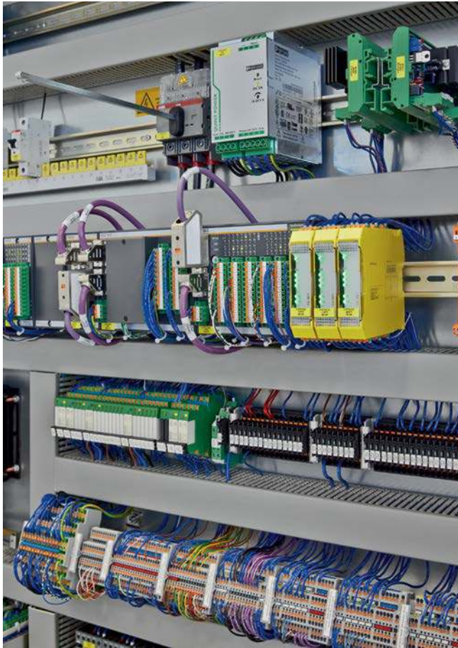
Figure 1: To automate its new selective-soldering systems, Ersä relies on multifunctional safety relays, as well as many additional components from Phoenix Contact.
